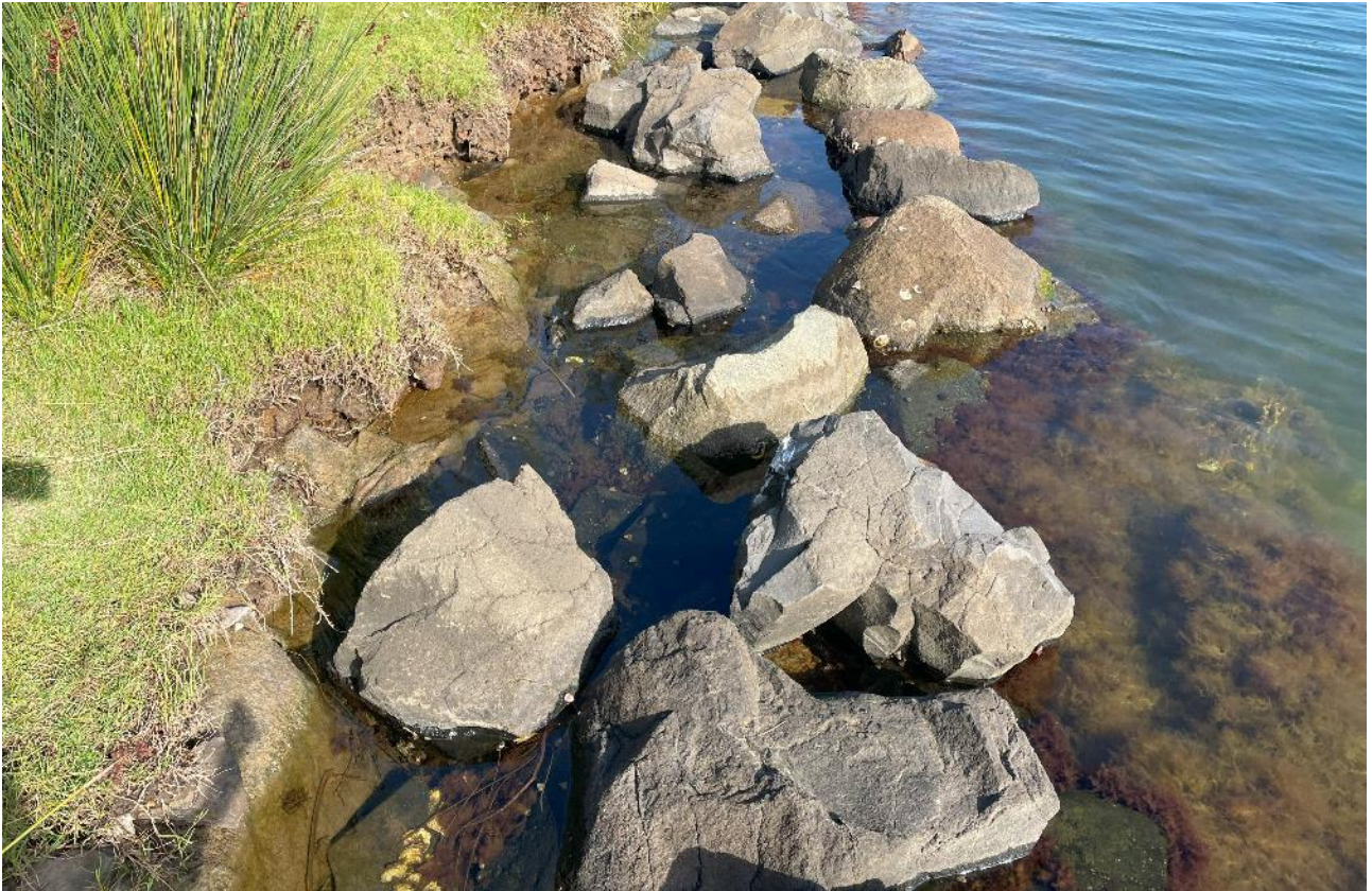
Figure 3-4 Ineffective Foreshore Rock Protection
