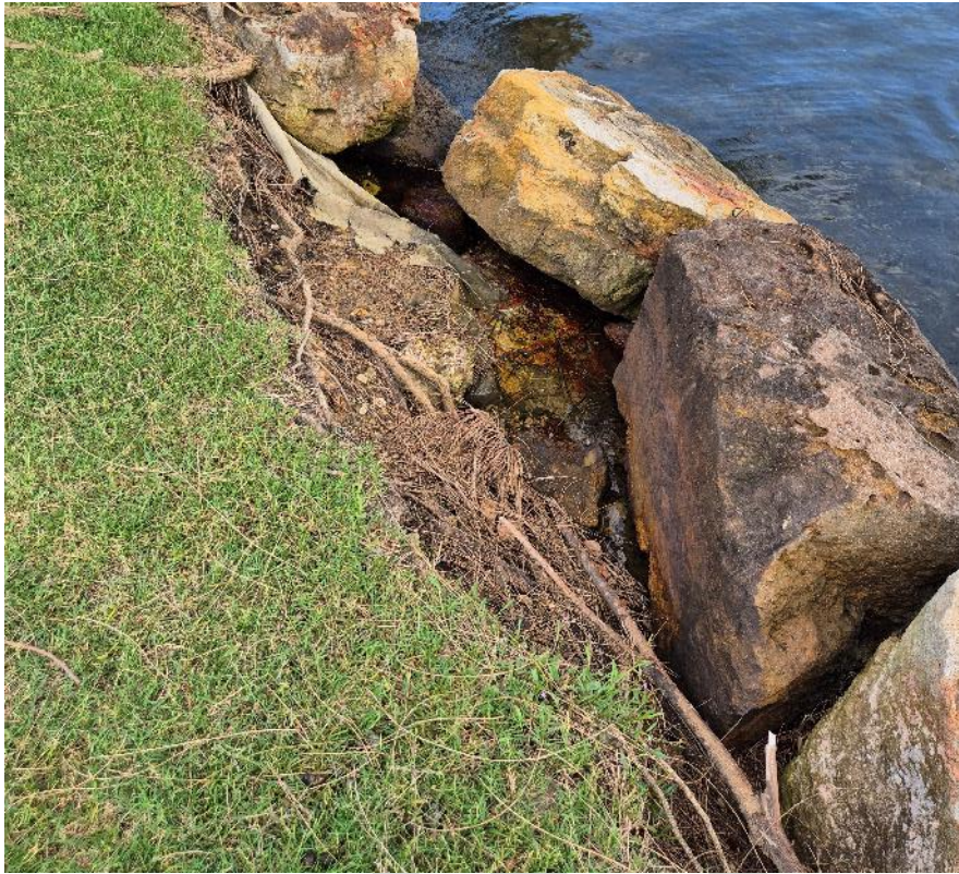
Figure 3-7 Rocks collapsed into the lake
