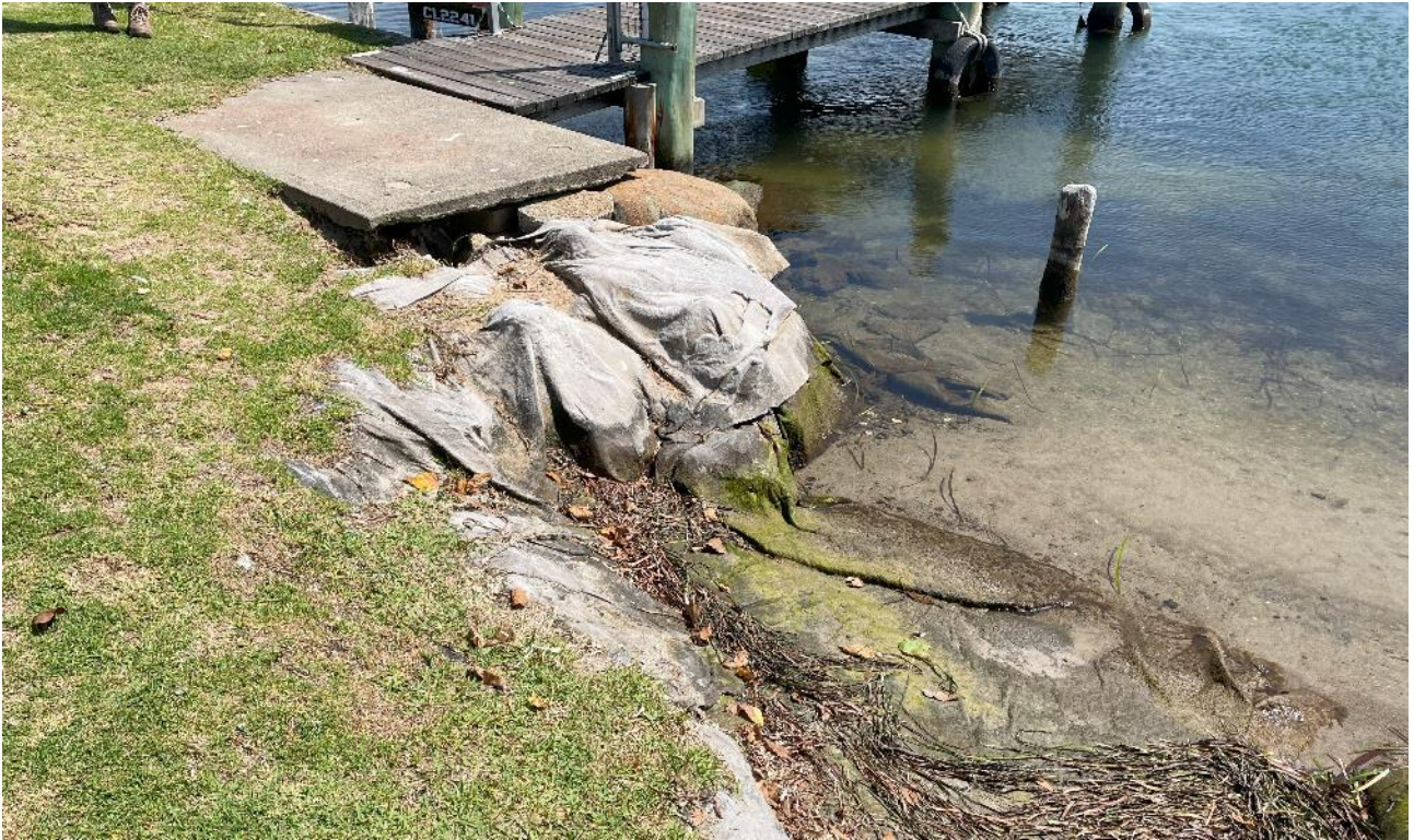
Figure 5-3 Undermined concrete slab and failed geotextiles on an eroding bank
