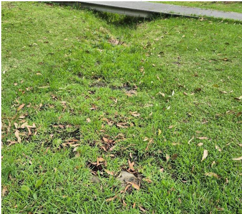
Figure 6-11 Drainage line infilled with rocks (looking downstream)
