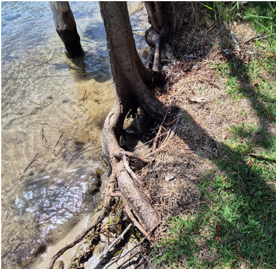
Figure 5-2 Exposed tree roots at the edge of the foreshore bank
