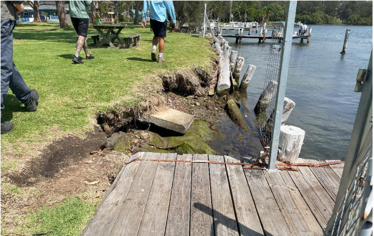
Figure 5-5 Foreshore erosion and failed log revetment
