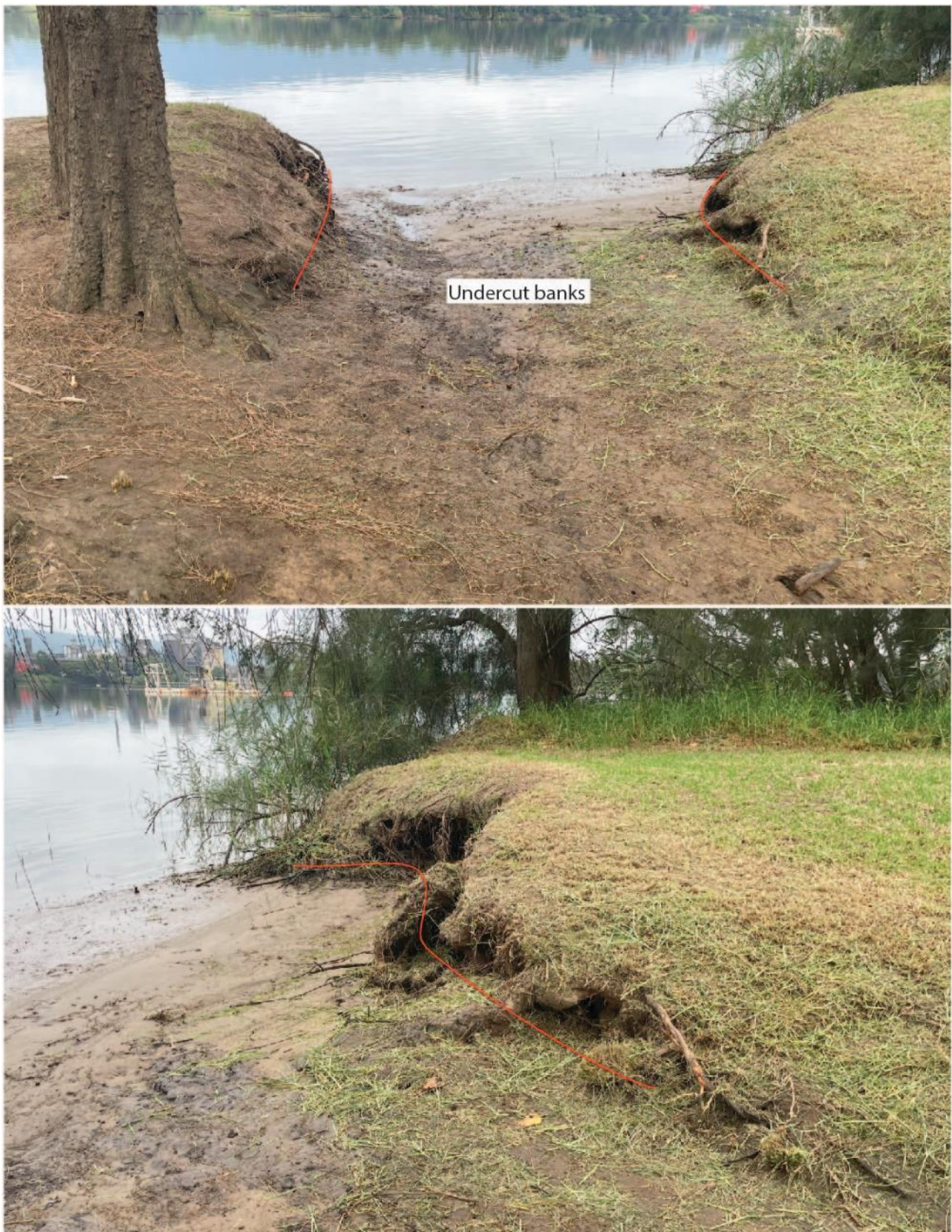
Figure 7-3 Stormwater outlet eroding at riverbank
