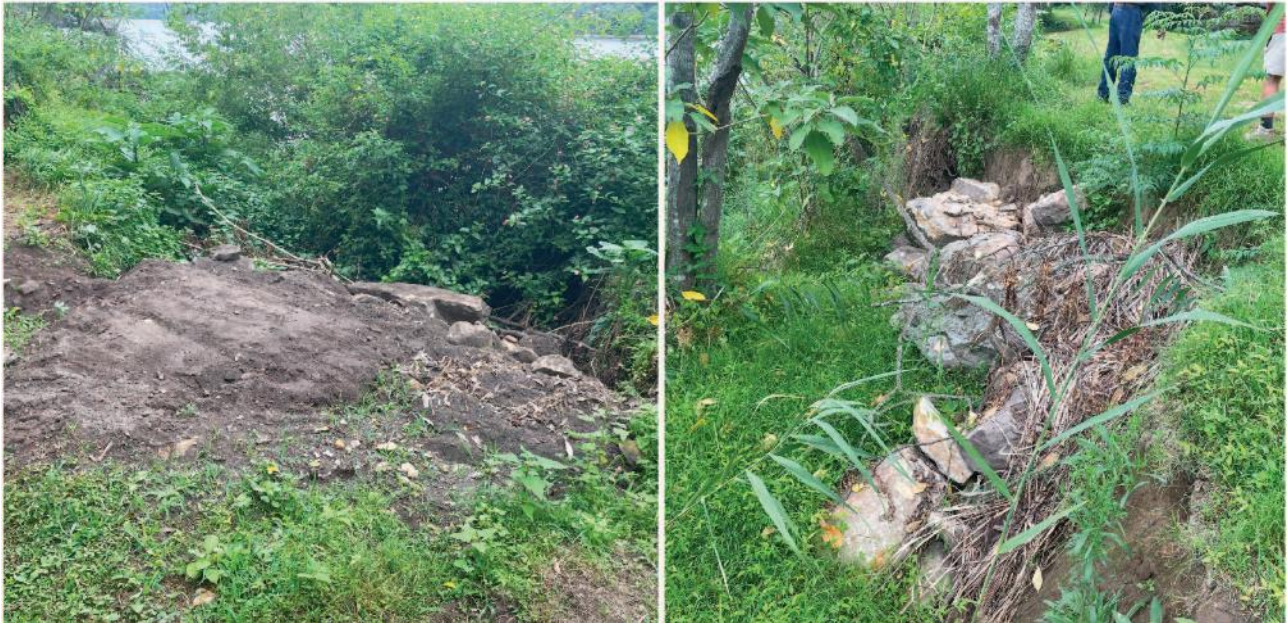
Figure 4-3 Informal works to treat erosion.
