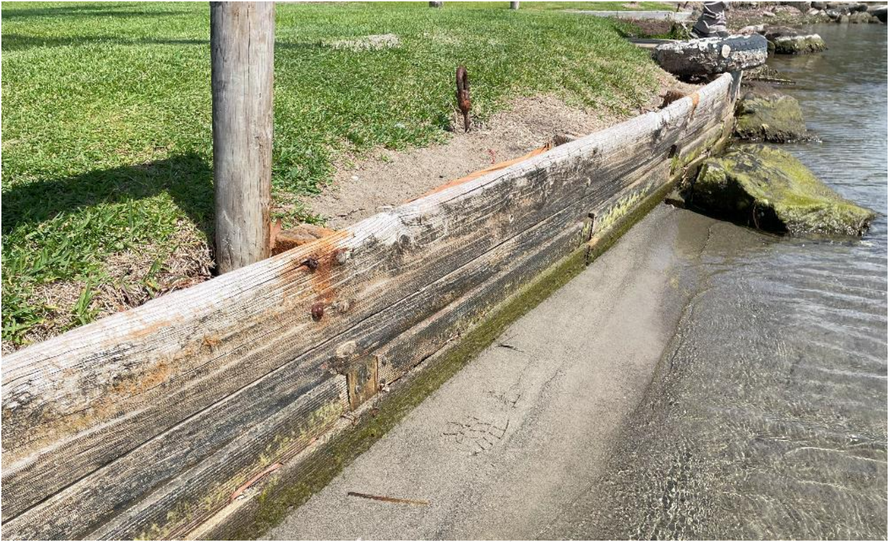
Figure 5-7 Scouring behind wood revetment
